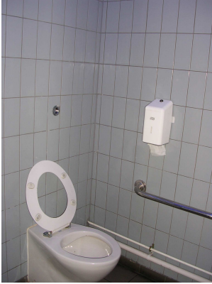
Many accessible toilets have poor fittings and fixtures.
